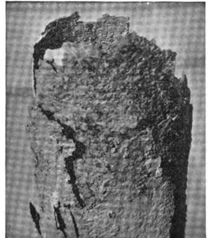
Fig. 4—Steel, Showing Aggravated but Typical Corrosion Resulting in Flaking or Scaling.
