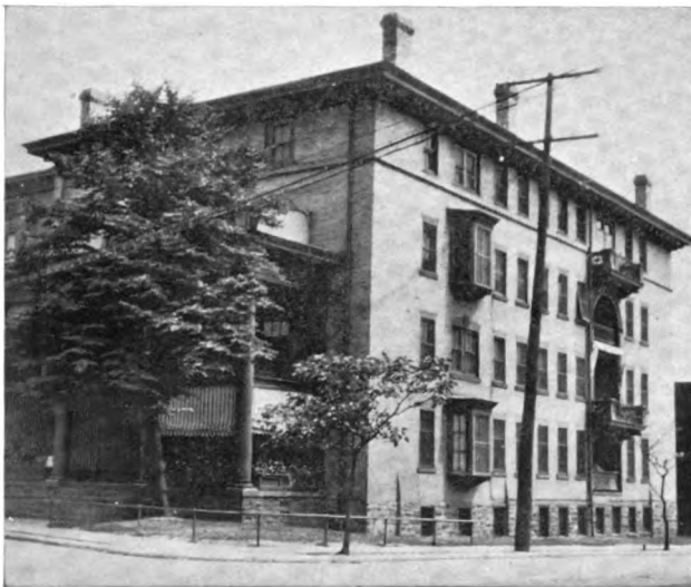
Kennett Apartments, erected 1902, equipped with brass pipe. Record No. 4, page 13. Typical of most apartments equipped with brass pipe, the hot water mains being badly corroded after 10 to 15 years' service.
