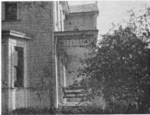
Home of D. E. Eakin, Allegheny County, Pa., erected 25 years ago. Part of an old galvanized iron rain leader, now from 50 to 75 years old, and taken from the old home when torn down, may still be seen in service at this place, while the new rain leader, seen at the corner of the house in above picture, has been renewed twice since the house was built, notwithstanding several paintings.
