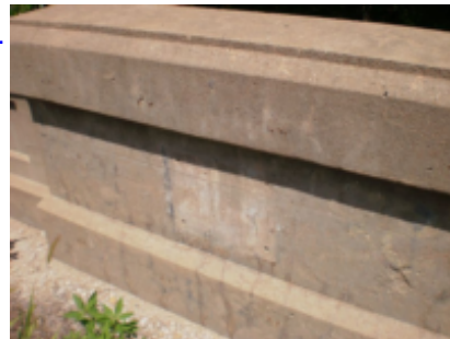
Rock Creek Bridge. Missing plaque on northeast wing wall. KRingler. 7-30-09
