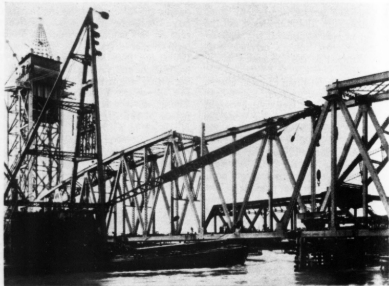
FIG. 8—DERRICK-BOAT ERECTION of the closing members of the span eliminated the need for falsework in the navigation channel.
