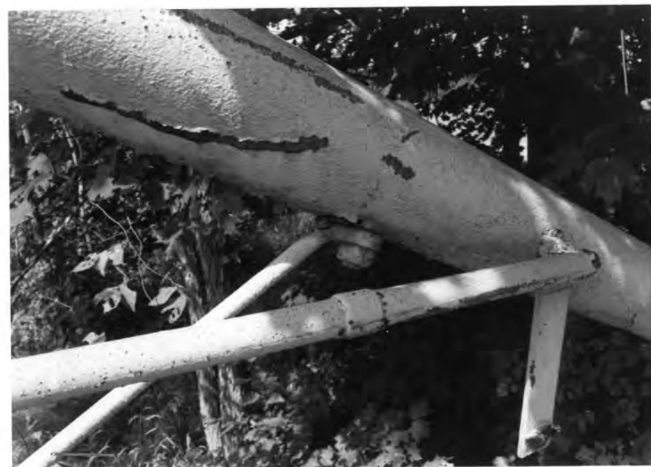
W TRUSS, N END, DIAGONAL CONNECTION TO INCLINED END POST, FROM SE 9-7-89
