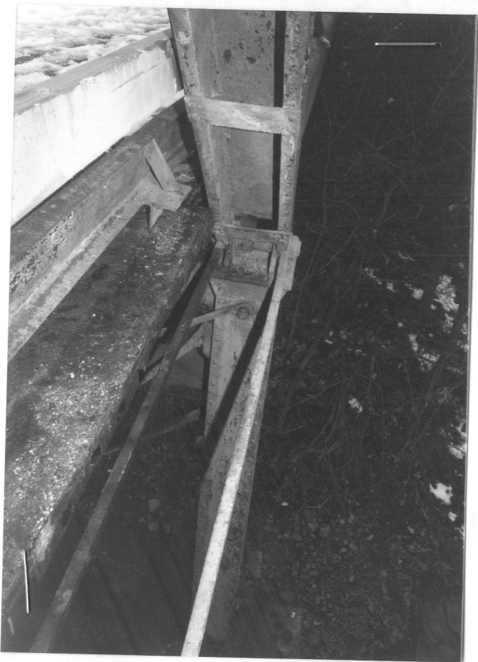
N TRUSS, W END, BEARING ON TOP OF POST ON PIER, FROM E (FLASH)
