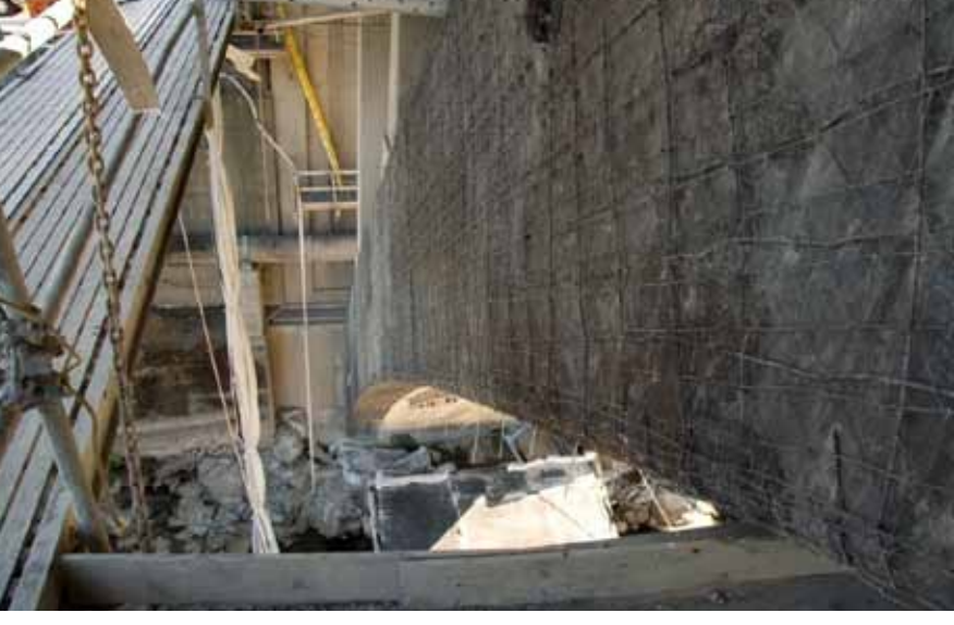
▼ Steel condition after Gunite removal
