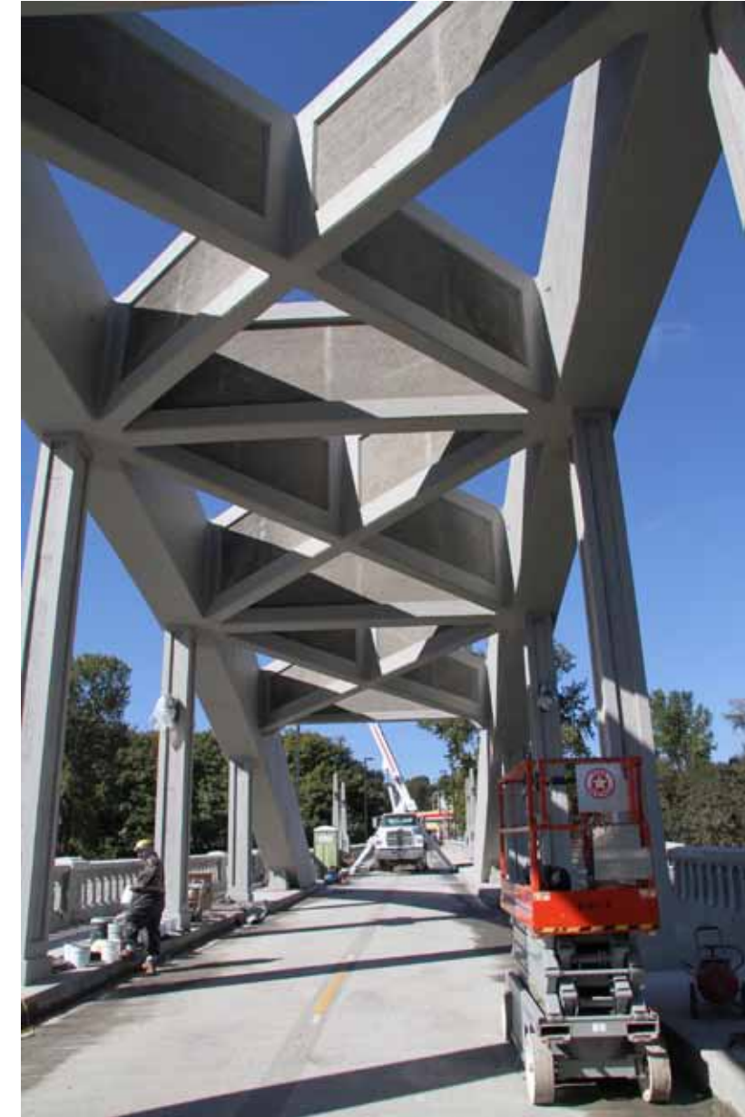
Concrete around the steel hangers was removed, damaged sections were plated and a new concrete encasement cast.
