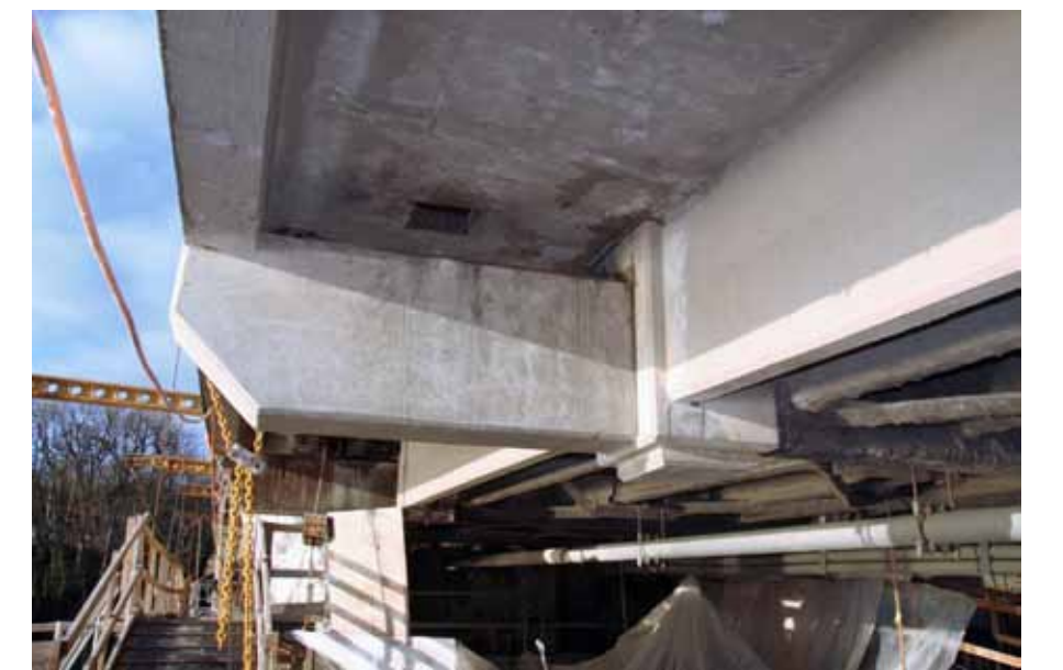
▲ Damaged floor beam extensions supporting the sidewalks were recast in new concrete.
