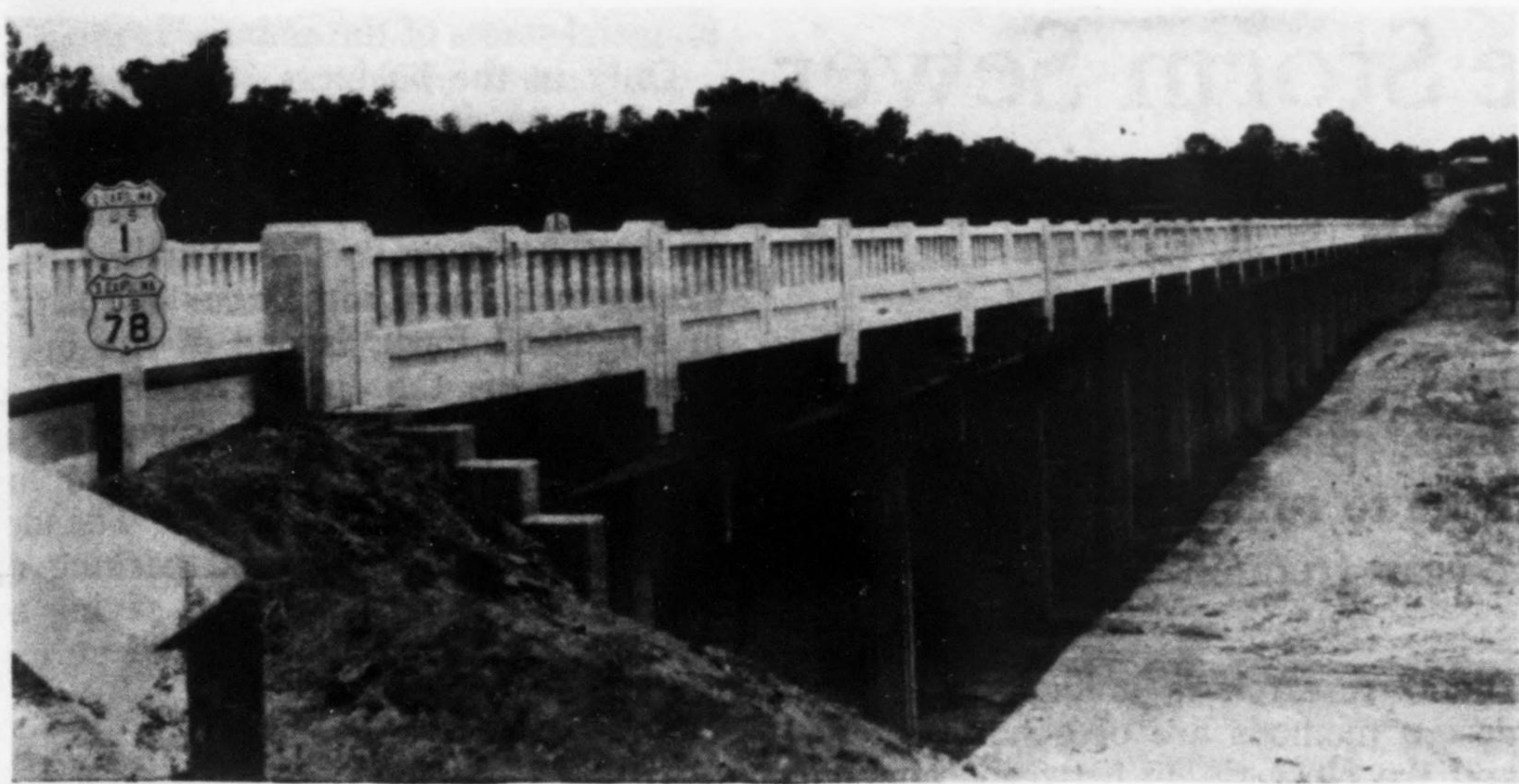
Fig. 4—Relief bridge of concrete deck girders that replaced 1,200 ft. of fill in approach to Fifth St. bridge, Augusta, Ga.
