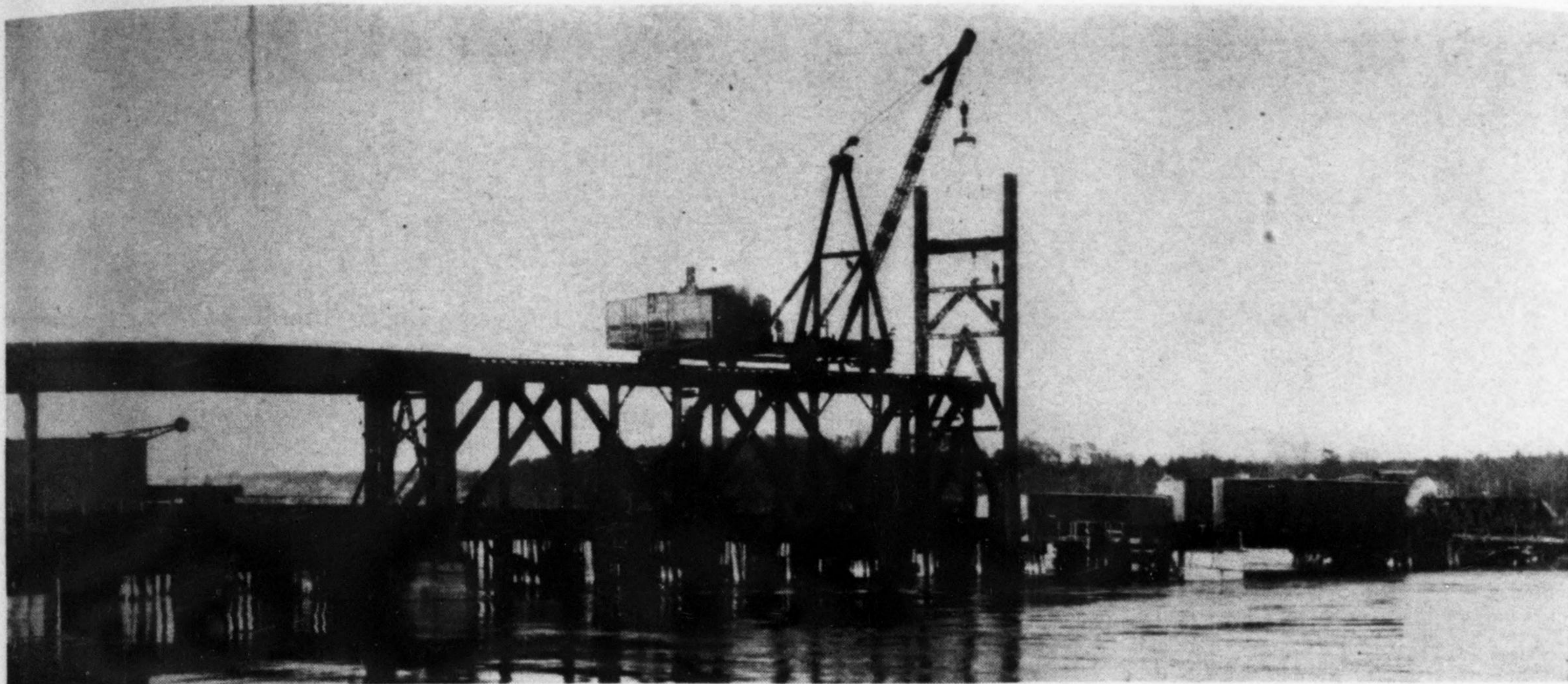
Lowering falsework bracing bent through whose hollow legs H-piles were driven to rock.
