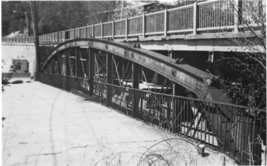
Figure 15. Lower Rollstone Street, Fitchburg, Massachusetts. The cast-iron washers for the ends of the web diagonals and the rather short segments of the top chord can be seen as well (bottom right) as the ornamental casting that carried the fabricator's name. Photo by author, 1995.
