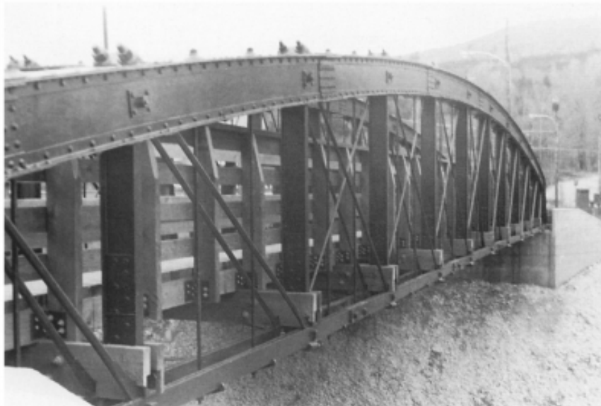
Figure 13. The Northfield bridge refurbished and carrying the Vine Street sidewalk over the railroad tracks. The vertical hangers between the panel points, the double bottom chords, and their single-bolt splices show clearly. Photo by author, 1991.
