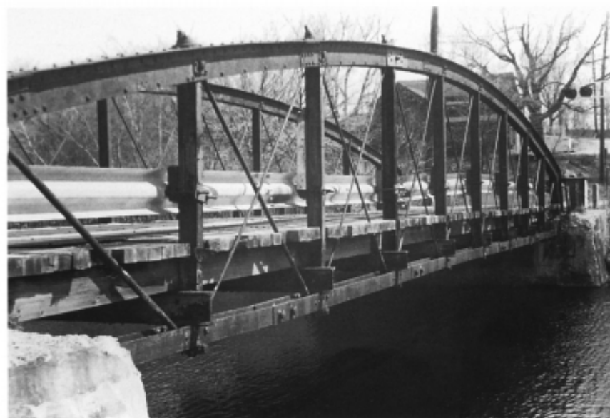
Figure 17. Webster, Massachusetts, at its original location. The short segments of the top chord, bottom-chord connections, and splices are all evident. Photo by author, 1997.
