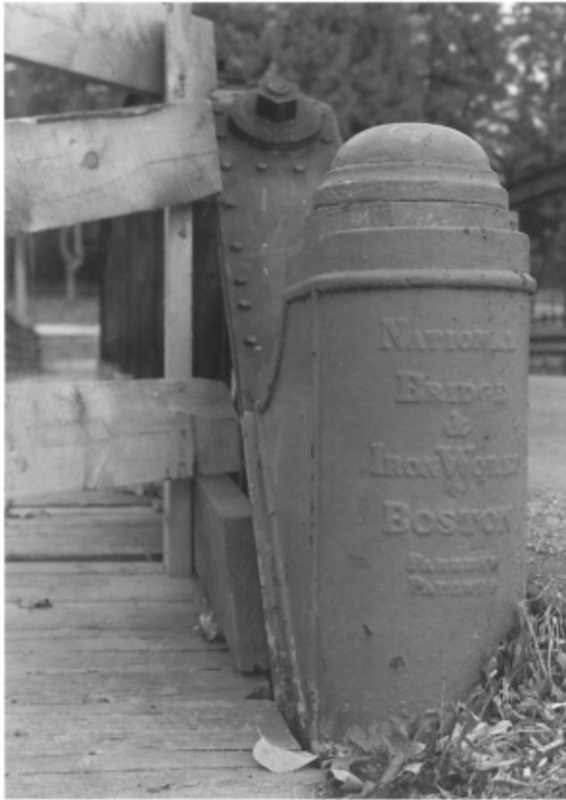
Figure 22. The ornamental casting, obviously an extra, that National Bridge and Iron Works installed on a few bridges. It also protects the end post from vehicles. Woodstock, pictured here, and Fitchburg have them. Courtesy of HAER Collection, Library of Congress, VT3-21, 803128.
