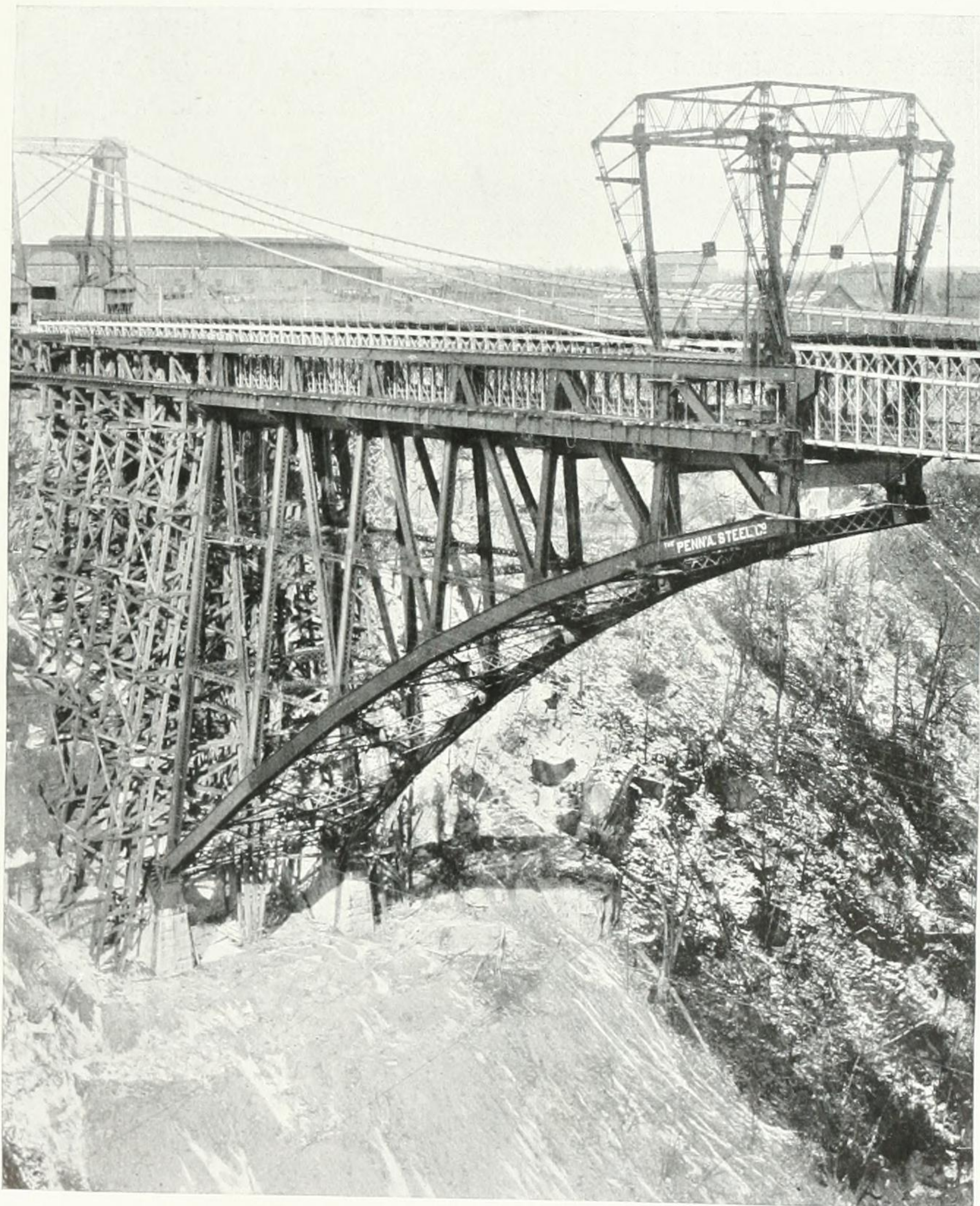
BUILDING THE SINGLE-SPAN STEEL ARCH BRIDGE AROUND THE OLD SUSPENSION BRIDGE ACROSS NIAGARA'S GORGE.
